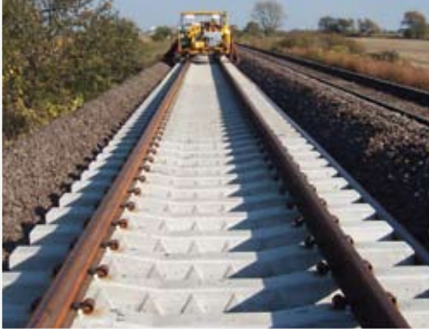
Tie used on a industrial line
